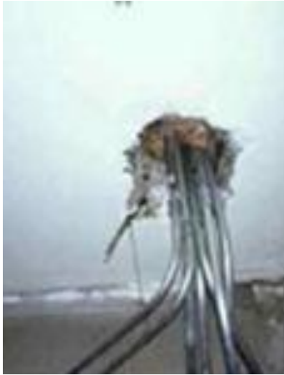
Wall penetration with no firestop
