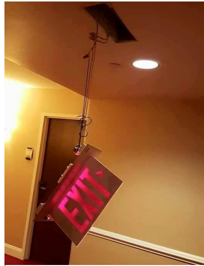
Exit sign inoperable or broken
