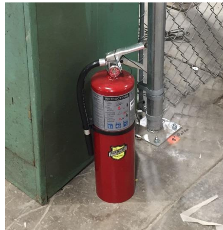
Fire extinguishers shall be installed on approved hooks and will be certified annually with a current tag
