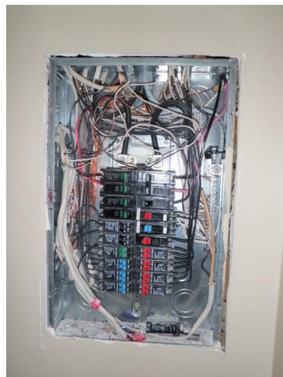
Open electrical panel
