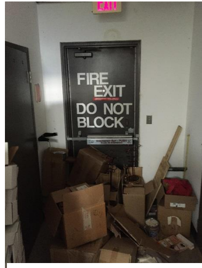
Blocked Exit and storage
